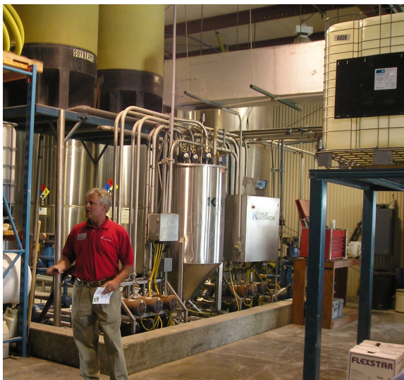
Bill Garver of Brandt Consolidated, Inc. explains their bulk pesticide containment area at the 2006 AASA kickoff event in Ashland, IL.
